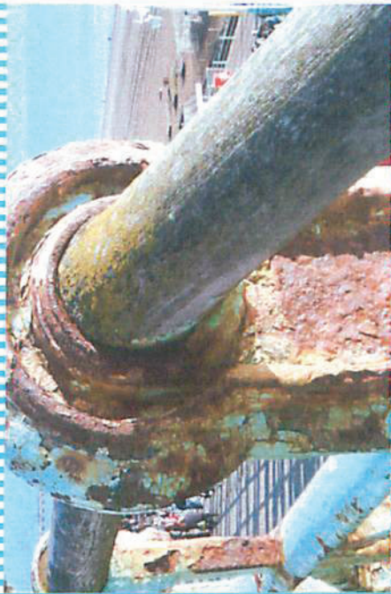
Seafront Railings Abandoned
